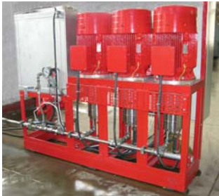
Booster Pump Water Mist, Water-driven Proportioning Fixed System
